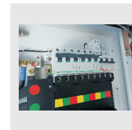
Theree Phase MCB Enclosure with Main Switch Space
